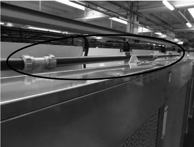
Ramp piping view
