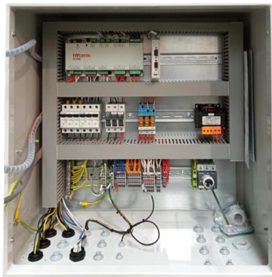
Q2Y - Electrical panel for EC fans
