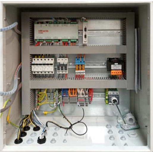
Q2Y - Electrical panel for EC fans
